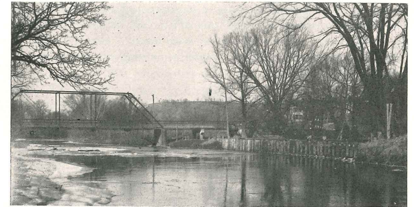
A stream meander was beginning to undermine bridge abutment. The string of piles ended the threat.
